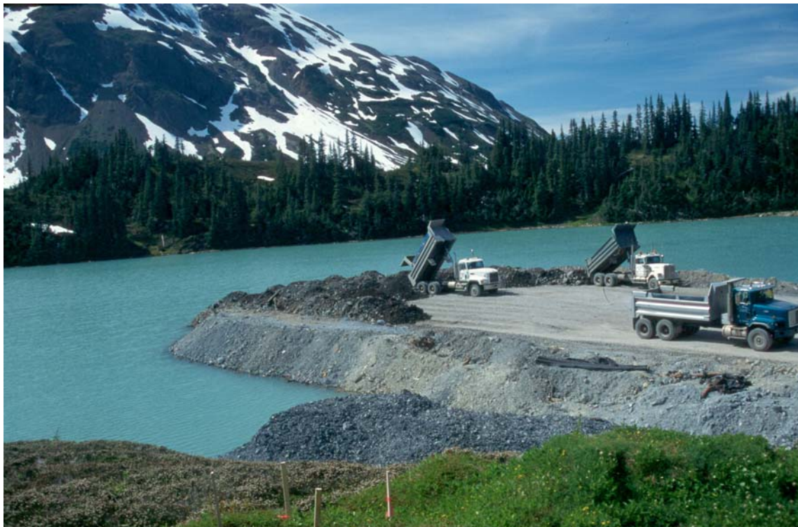
Figure 1-2. Photograph of the relocation and submergence of ARD-releasing waste rock shown in Figure 1-1.
